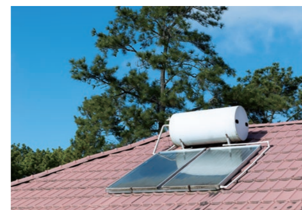
Solar heat collection panel
