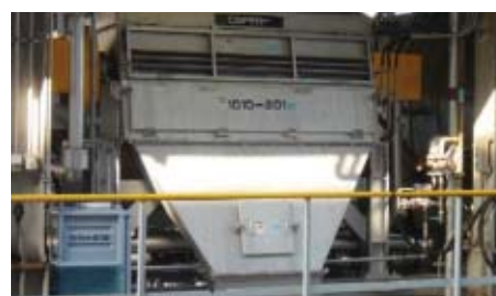
Effluent Condensing Equipment at Nagoya Factory
