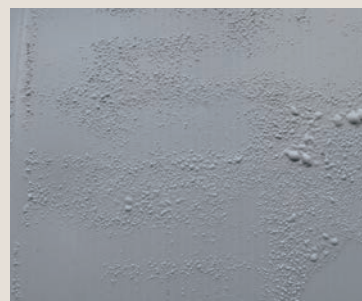
Photo 2 Coating film defects
