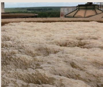
Photo 1 Reaction tank about to overflow
